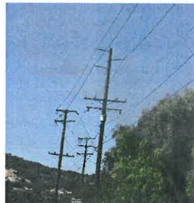
Example of overhead powerlines
