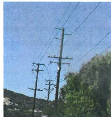
Example of overhead powerlines
