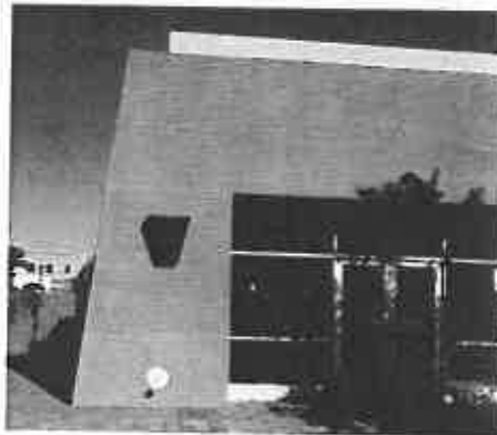
Horizontal banding in plaster
