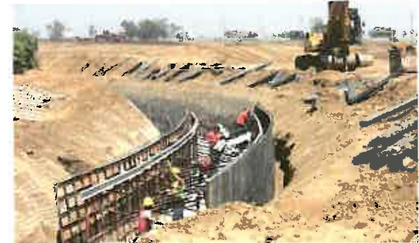
The RCFCWCD manages flood control projects such as the construction of the Nason Basin, above. In 2003, the District completed the construction of the 16-acre basin, which reduces the 100-year flows by more than 70%. Photo credit: RCFCWCD, rcflood.org
