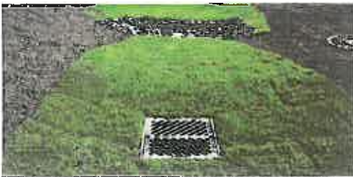
Infiltration trenches detain water for brief periods. This trench at Seattle-Tacoma Airport includes vegetation appropriate for an airport environment.
