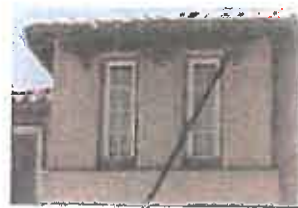
Exposed rafter tails
