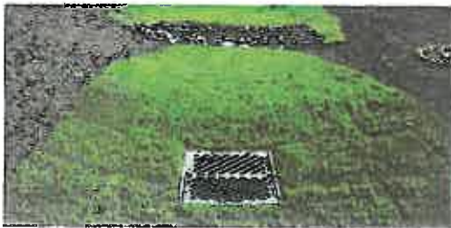
Infiltration trenches detain water for brief periods. This trench at Seattle-Tacoma Airport includes vegetation appropriate for an airport environment.
