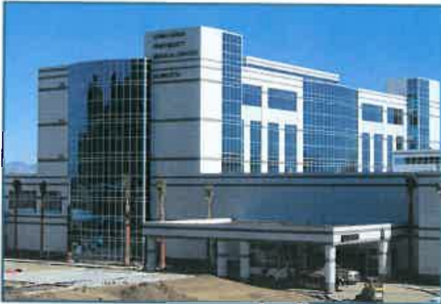
Shown here under construction in 2010, Loma Linda University Medical Center-Murrieta is a catalyst for growth in the North Murrieta Business
