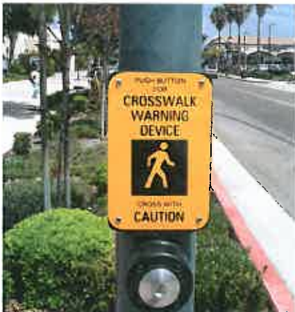
Crosswalk push button for pedestrian warning device
