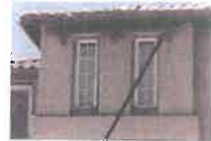
Exposed rafter tails
